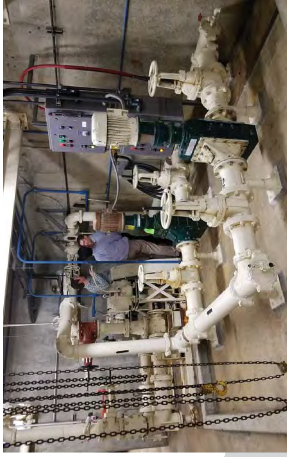
Primary sludge piping gallery at in-line grinder and pumping station.
