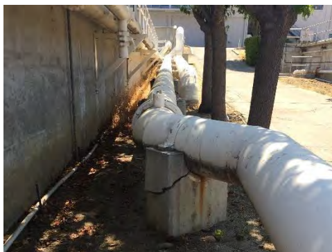
Left: Failing pipe support & coating needs
