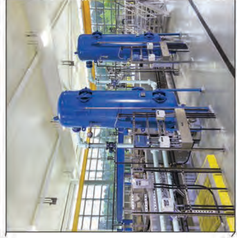
CLEAN AND SIMPLE PROCESS AREA
