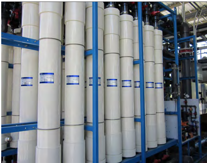
CDM Smith employed a semi-universal UF skid design for the San Diego Demonstration Plant to allow testing of alternative membranes on a single skid
