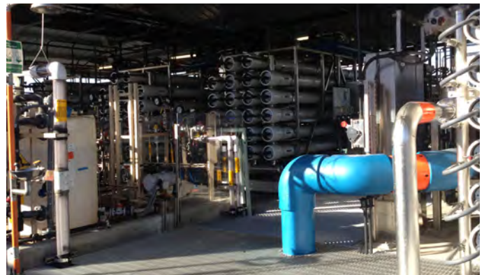
The brine recovery system for the Vander Lans WTF has been operating for two years achieving 92.5% RO recovery.
