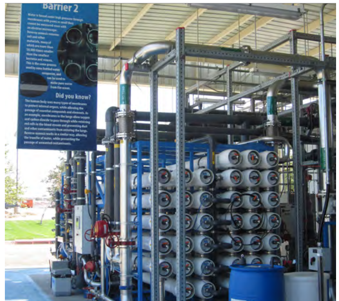
CDM Smith-designed demonstration project at San Diego includes education signs for public tours, to aid in building public support.
