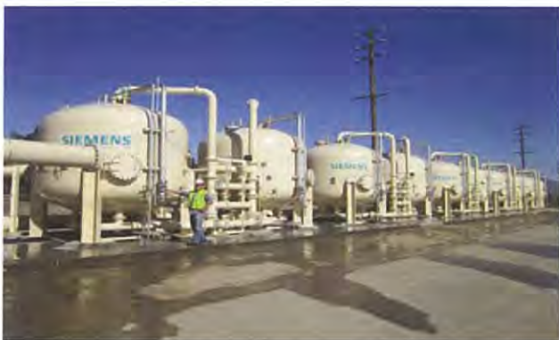
Figure 2: GAC Vessels at Tujunga Wellfield
