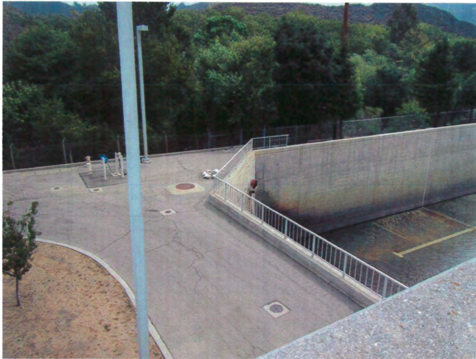
Figure 14 – Storm water pipe that drains into the balancing pond
