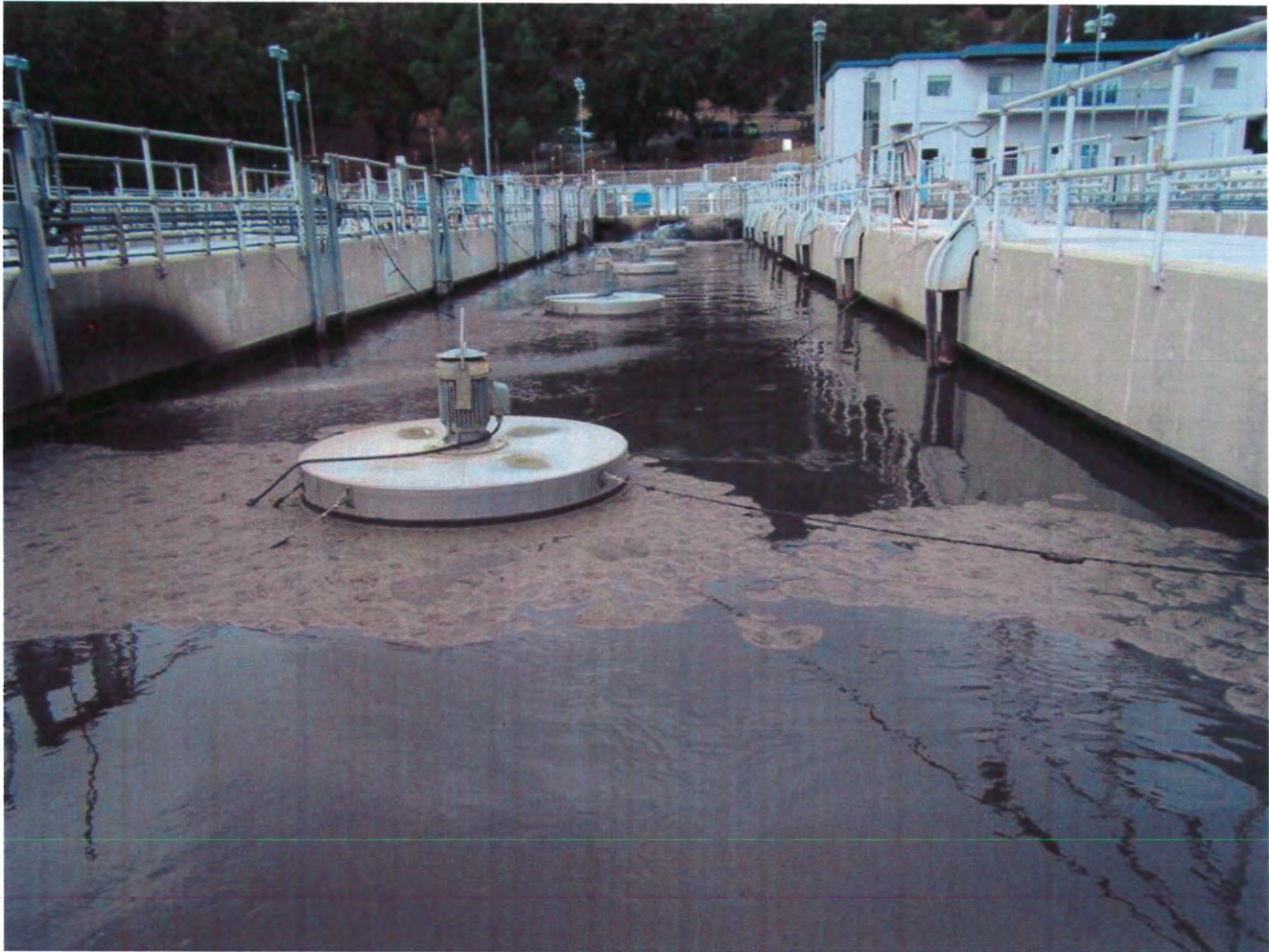
Figure 7 – Biological Nutrient Reduction Units No. 3 (Anoxic Zone)
