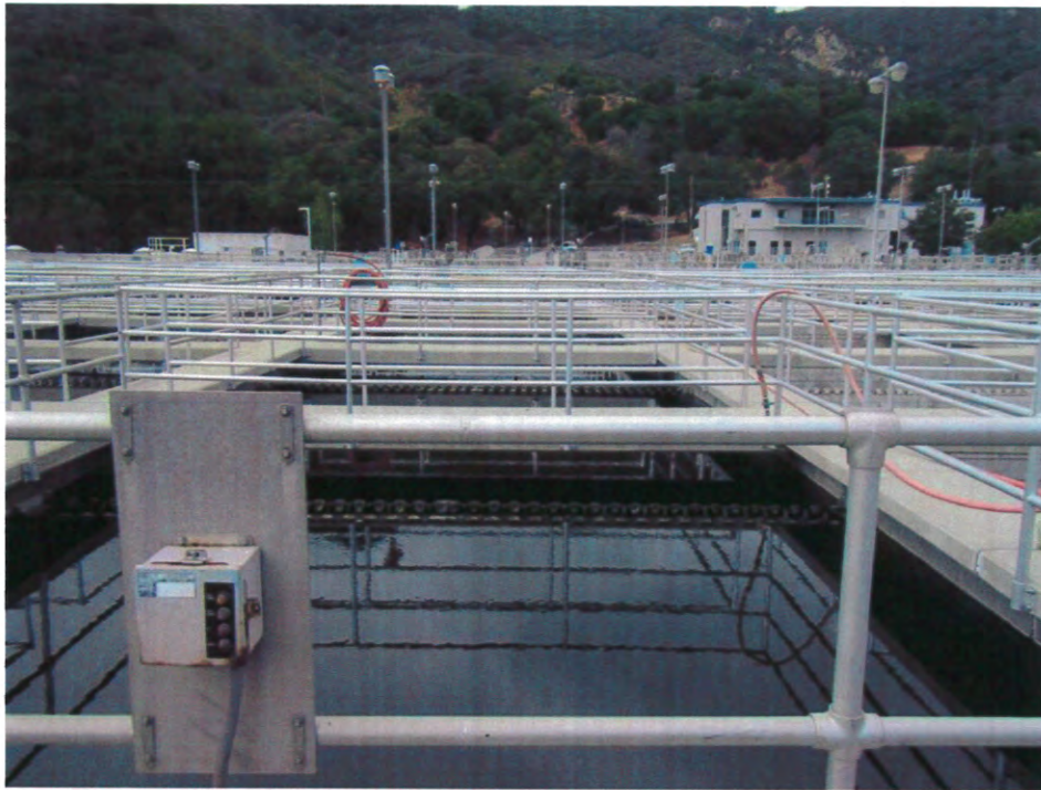
Figure 10 – Wastewater at the end of a secondary clarifier
