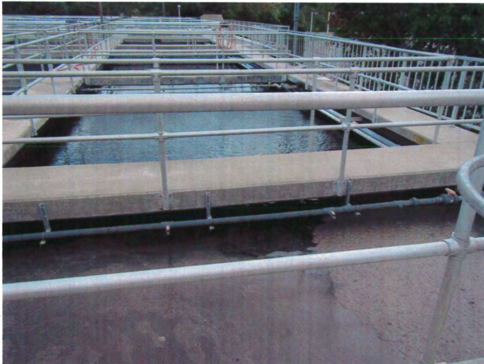
Figure 9 – Wastewater entering a secondary clarifier
