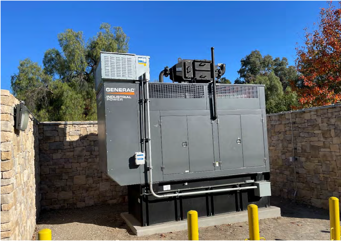
Figure 1- 200 kW generator installed at Jed Smith Pump Station
