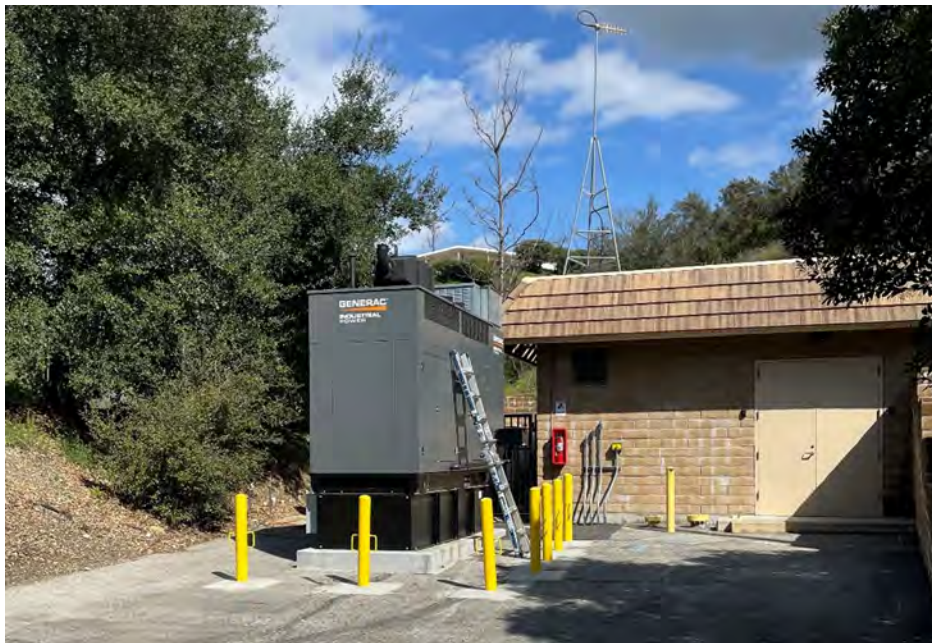
Figure 2 – 200 kW generator at Cold Canyon Pump Station
