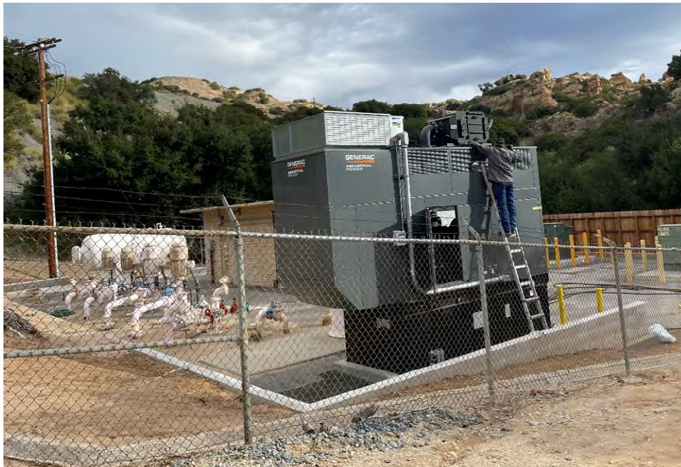
Figure 4 - Preparing for Load Bank Test of 500 kW generator at Twin Lakes Pump Station
