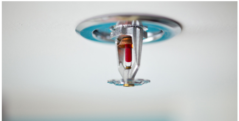
Homes built during and after the 1990s typically have fire suppression systems (sprinklers) as part of building code requirements.
