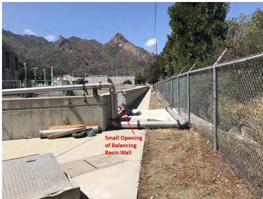
Photo of the Balancing Basin Wall and the Small Opening (Looking west or upstream)
