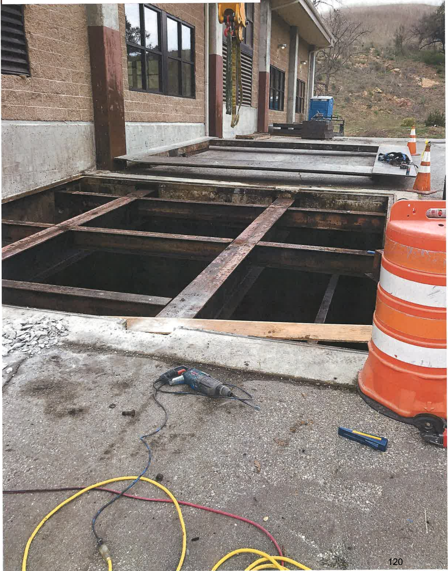
(Before) Grizzly Plate Structural Beams Fire Damage
