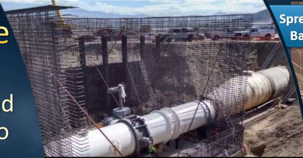
Added new interconnections and strengthened existing infrastructure to enable DVL water to be delivered to Mills
