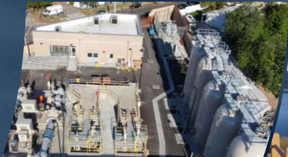
Rehabilitated Greg Ave. Pump Station for improved reliability of Colorado River water to the SWP Dependent Area
