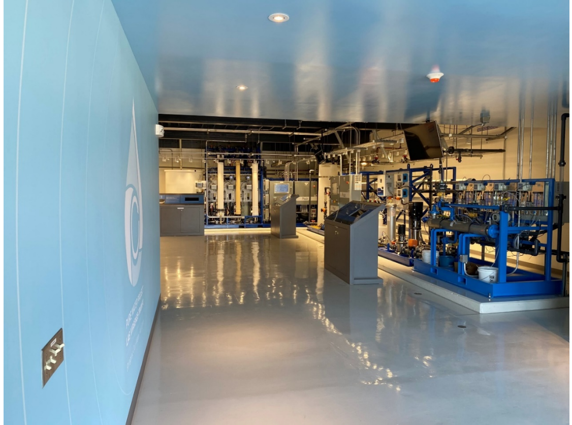
Figure 2 Interior of LVMWD Pure Water Demonstration Facility.
