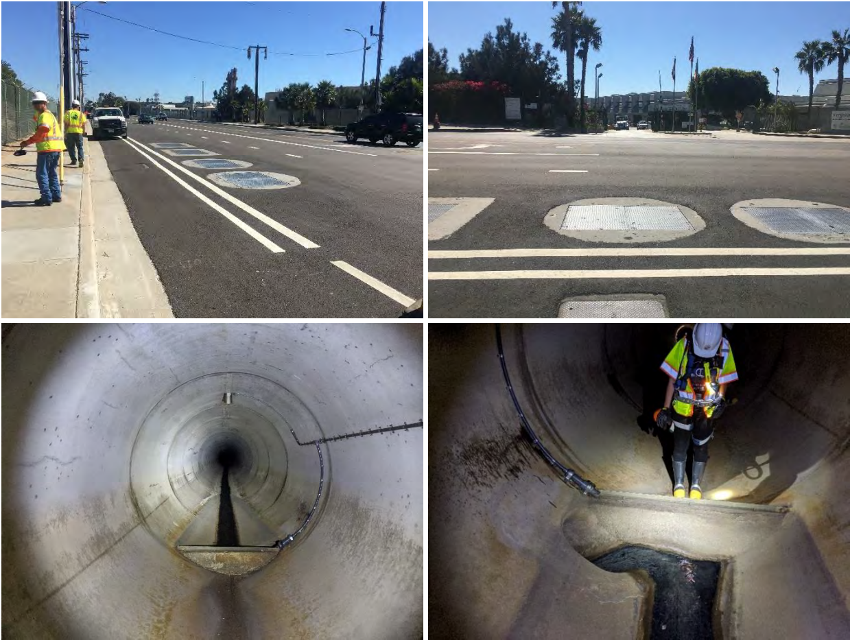
Photo 3-1. Pershing Drive DWD; Photographs taken during October 22, 2019 Site Visit with LACFCD Staff
