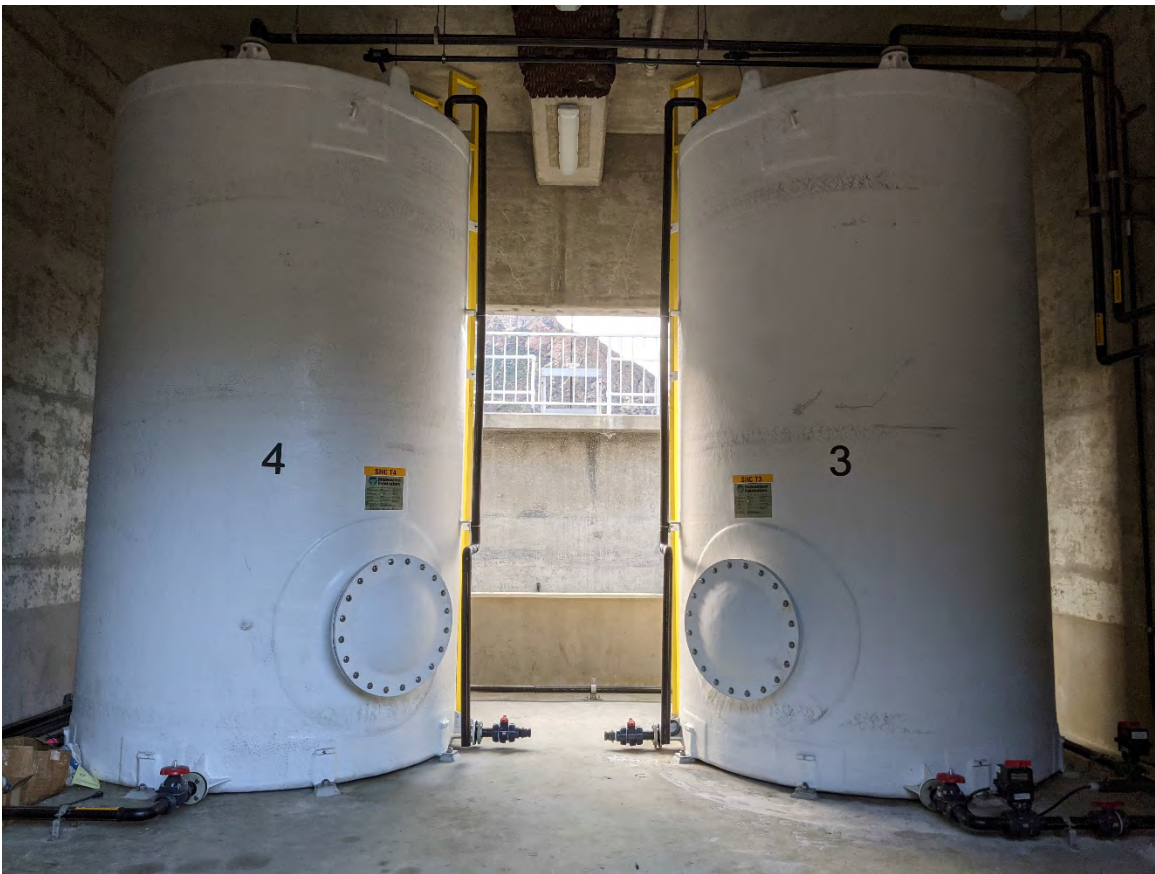
Figure 2: Upper Chemical Room Tanks 3 and 4
