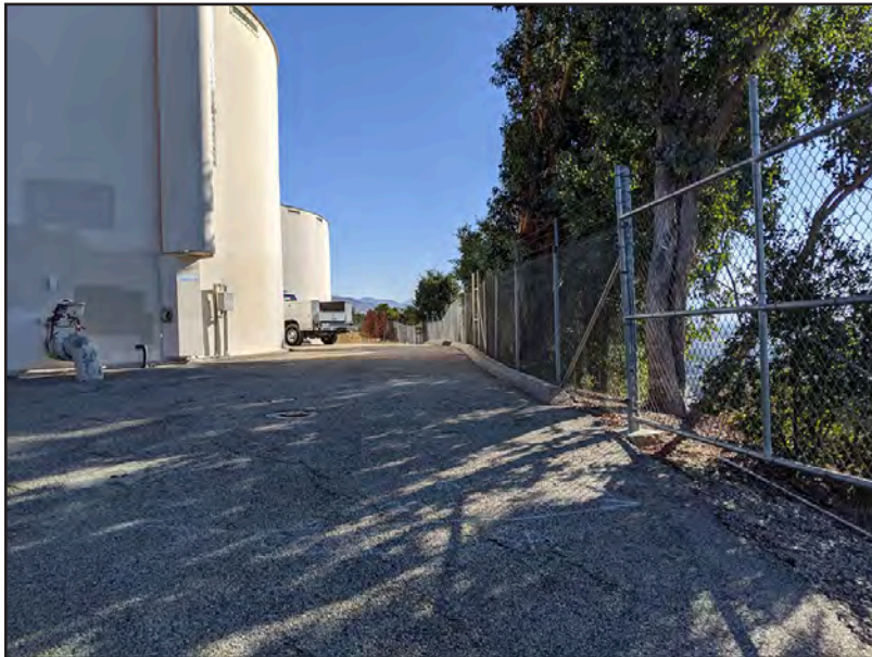
Photo 1A – View of the south-facing side of the water tank to be replaced (left) and trees surrounding the paved area (right).
