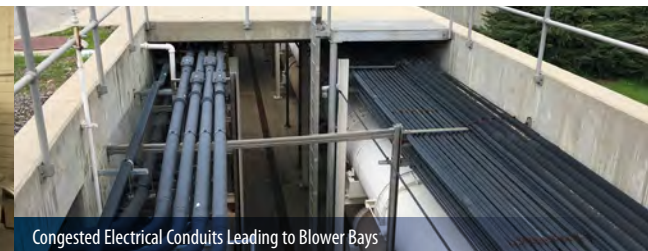
Congested Electrical Conduits Leading to Blower Bays
