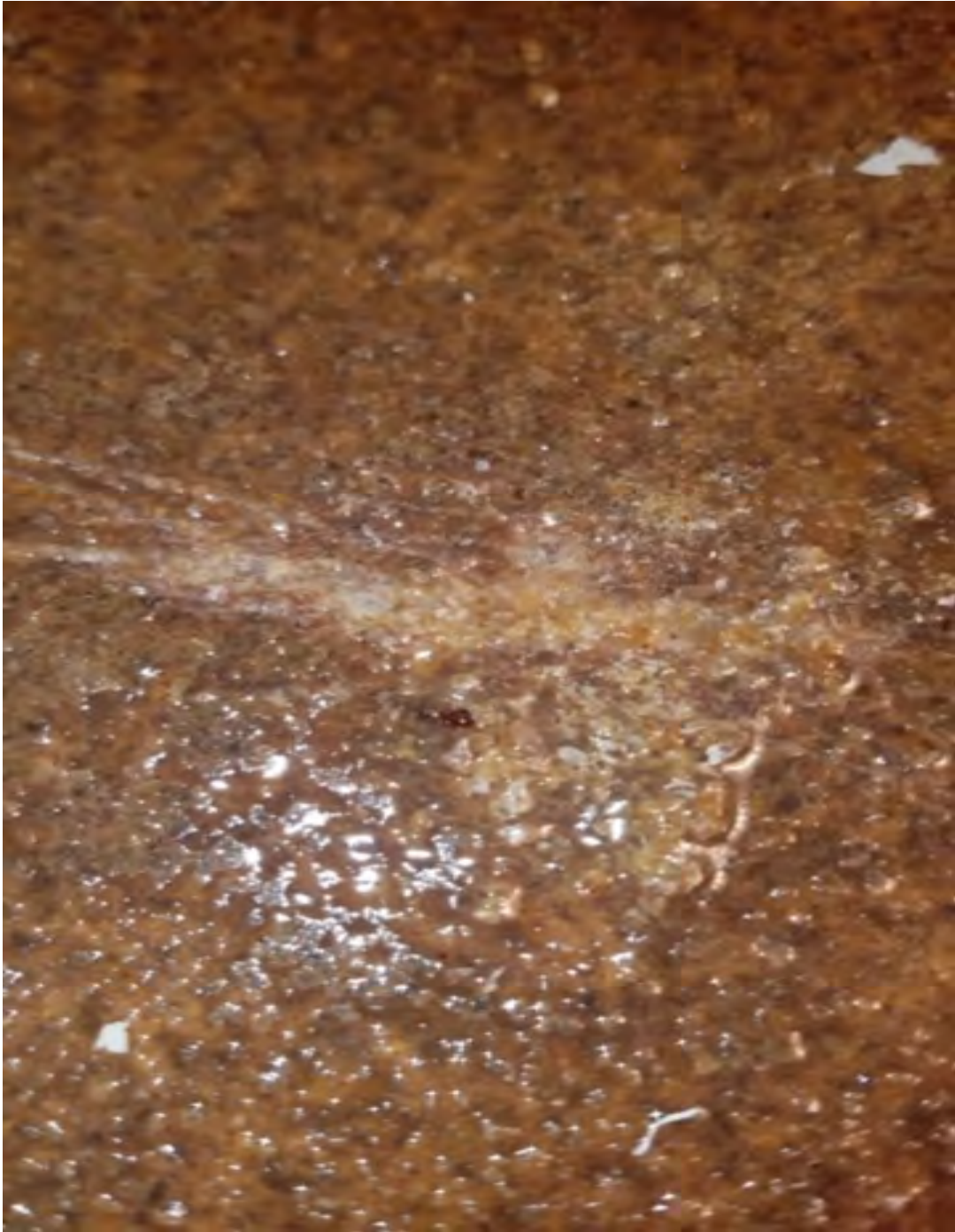
Grainy surface due to chemical deteriorating the coating
