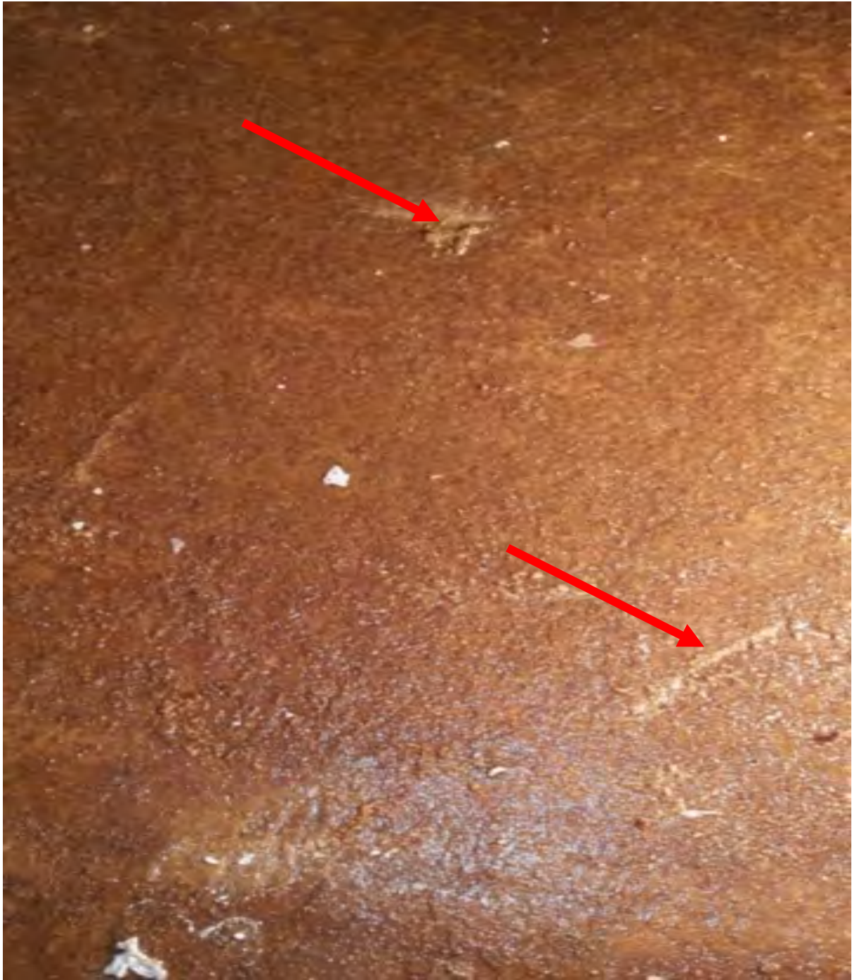
The surface of the inside of the tank show where the coating is easily coming off
