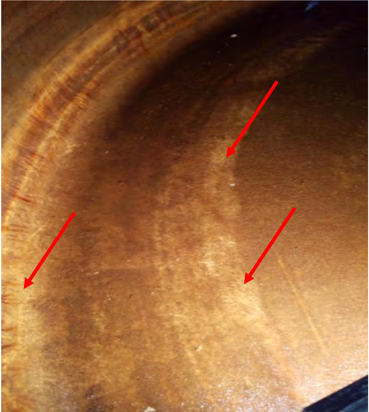
This picture shows the area in which the fiberglass mesh is starting to become exposed and there is near to no coating
