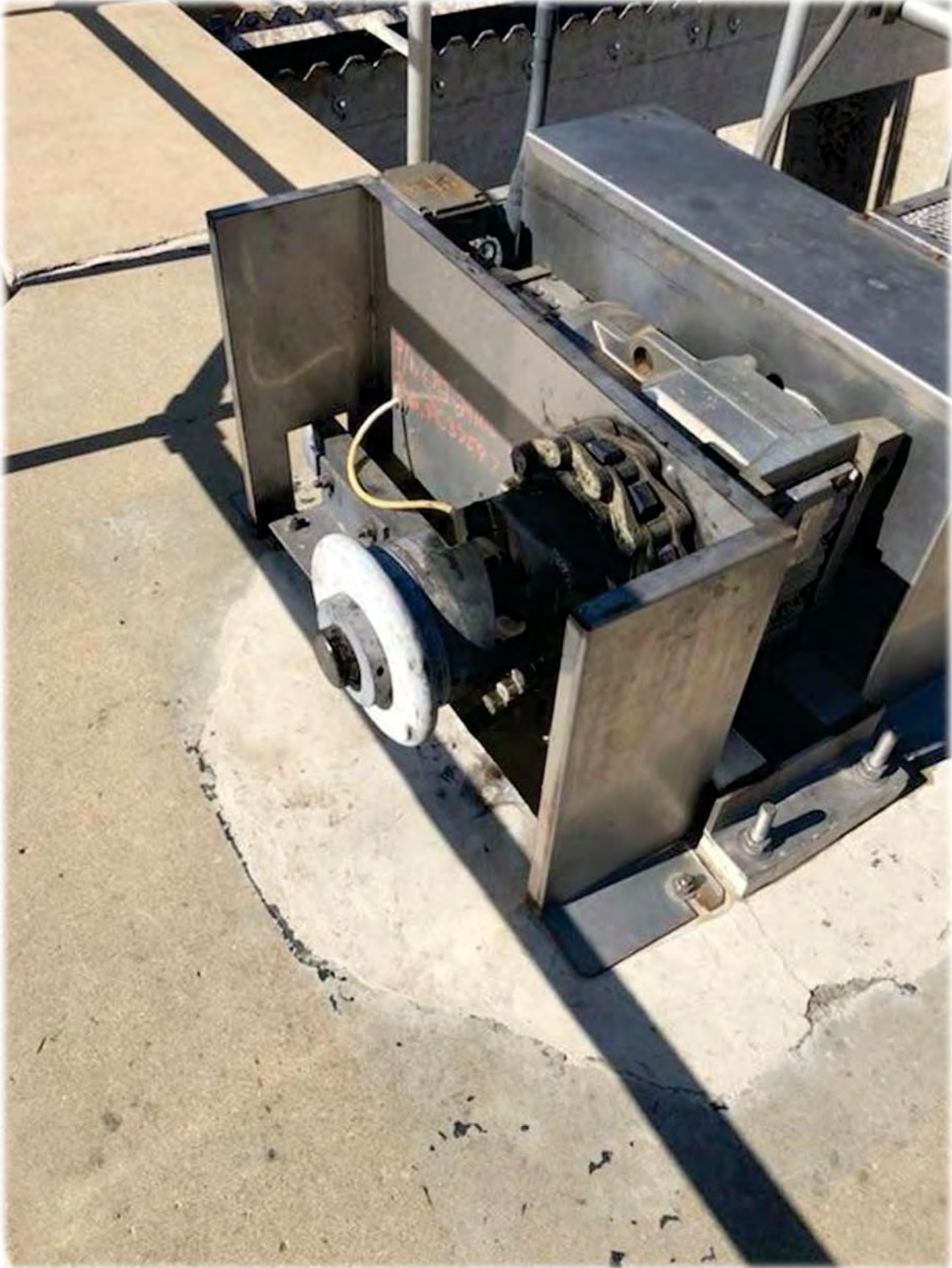
Existing Jaw Clutch System for Secondary Sludge Collection System Drive
