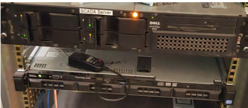
Figure 2-3 – Water Operations SCADA server rack with external modem
